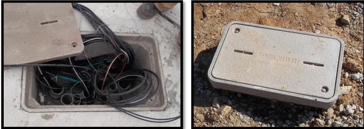
Exhibit 5-20 Junction Box in Concrete and Dirt
